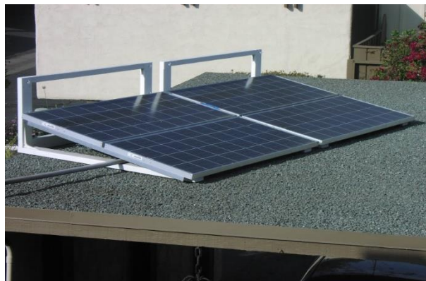
The level of solar radiation directly affects the power of the panel.
